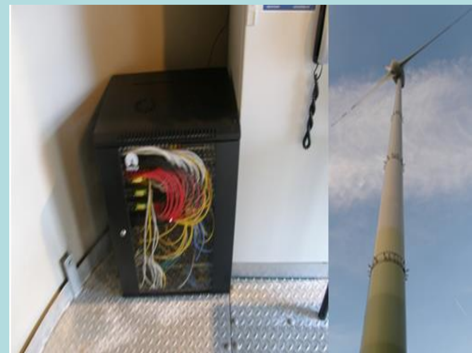
Fig. 2. B-finder unit: left - internal rack cabin, right - external sensors.
