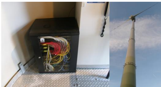
Fig. 1: B-finder unit: internal rack cabin and external sensors.
